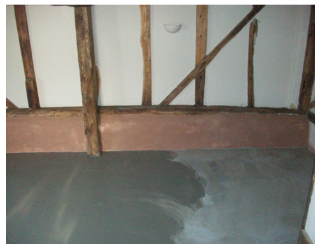
New internal rendering was made water and salt resistant by the inclusion of Trimix 1. The new floor slab was water and gas proofed with a coat of TT Vapour Membrane before the screed was applied
