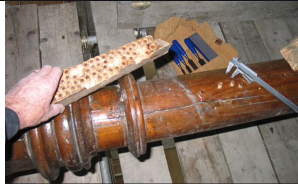
Preparation of 10mm pitch pine plugs for restoring drilled surface of exposed and ornate timbers injected with Tribor Gel
