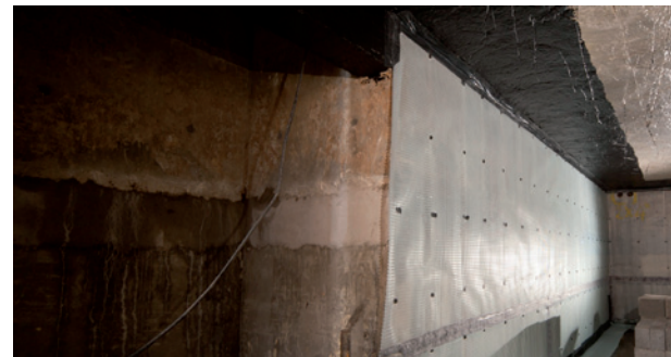
Triton TT Vapour Membrane was applied to the underside of the ground soffit and lapped 300mm down and behind the Platon cavity drain membrane to prevent and guide water migrating through the ground slab behind the wall membrane.
