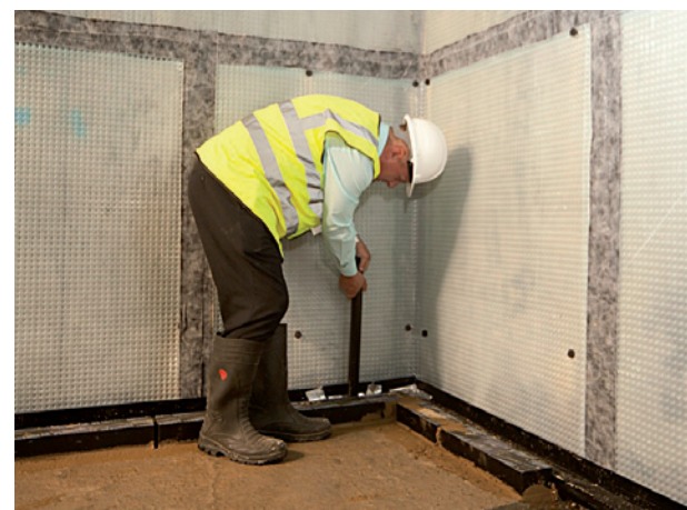
Installation of rodding eye extension to Aquachannel which will eventually protrude through block work for maintenance access purposes (close to sump pit which will house Aquapump Pro pump).
