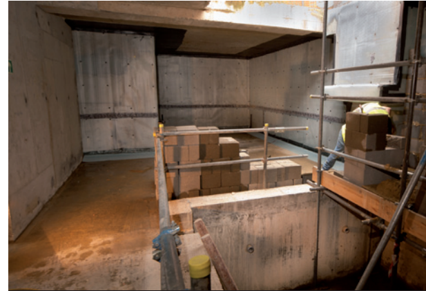
The complete below ground structure including the swimming pool was constructed using Triton's watertight concrete system.
