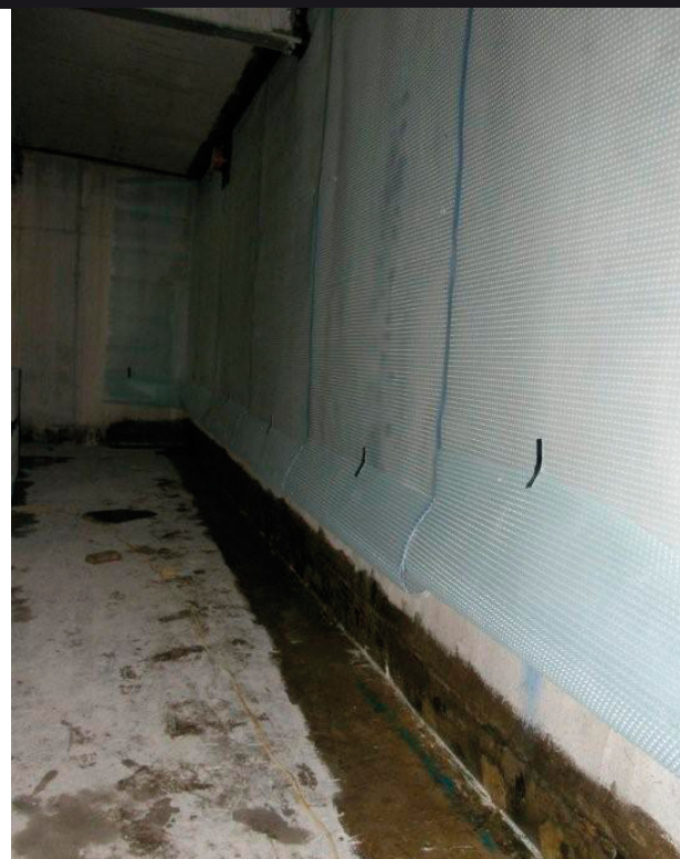
Reinforced concrete wall floor junction tanked with Trimol 40 epoxy resin, before installation of blockwork upstand to house Aqua Channel drainage detail
