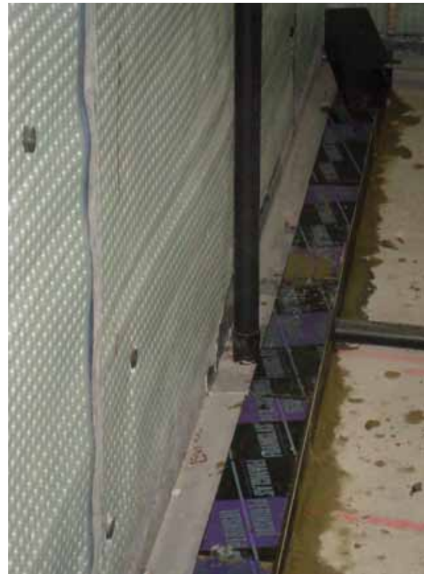
The cavity drain system in the upper basement lever was gravity drained down to the system below
