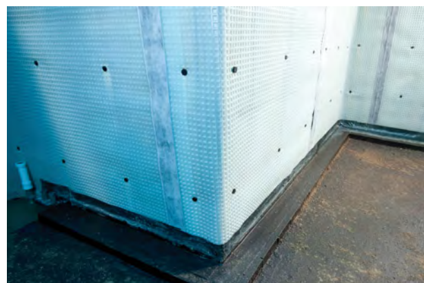
Engineering brick detail housing Aqua Channel, with non-return odour resistant valve awaiting fitting (far left)
